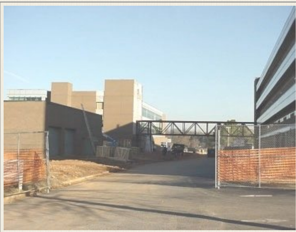
New lab space and autopsy area being constructed adjacent to GBI main building in 2002.
