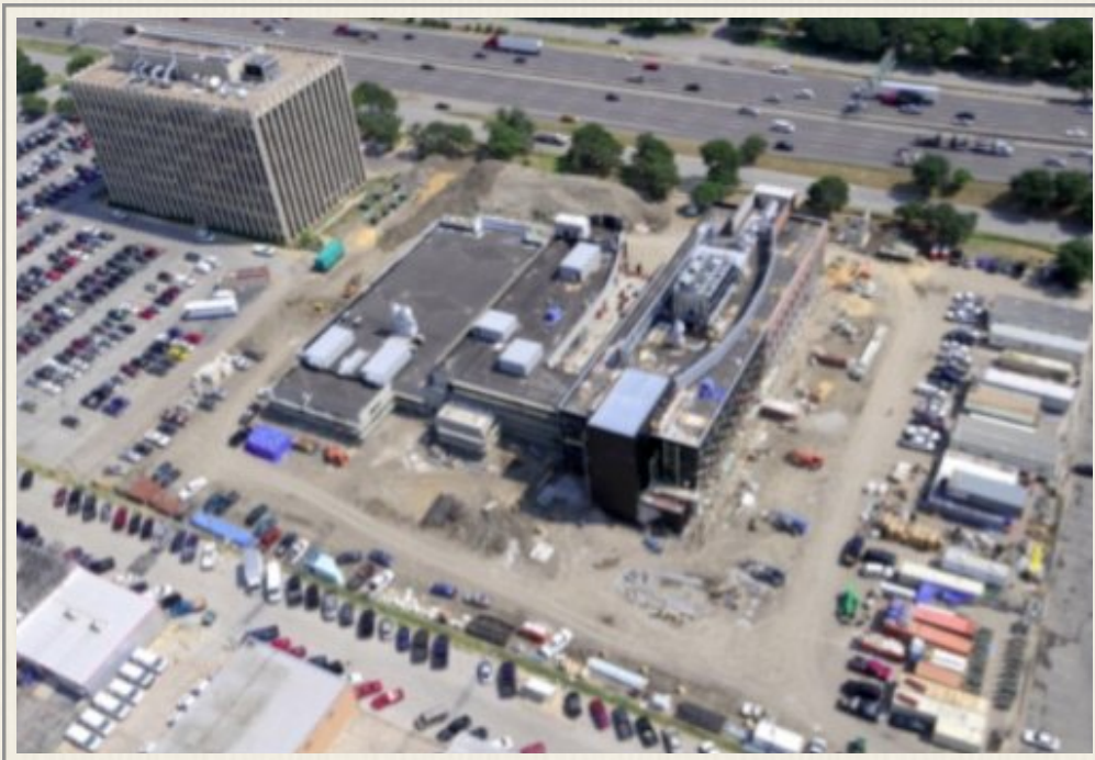
Aerial view of the construction of the new SWIFS 2355 N. Stemmons Freeway, Dallas, TX
