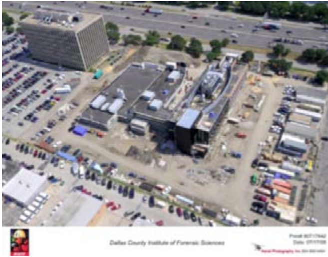
Aerial view of the construction of the new SWIFS 2355 N. Stemmons Freeway, Dallas, TX
